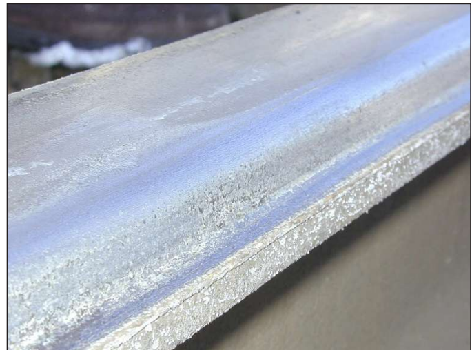
Figure 1. MBTA's shallow, 3/4-inch flange carved a shelf into the rail beneath the tip of the flange.
